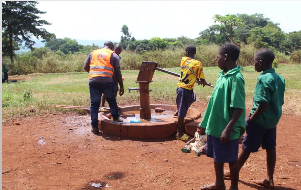
Poor hygiene of the borehole at Kinywamurara Primary School- Masindi District
