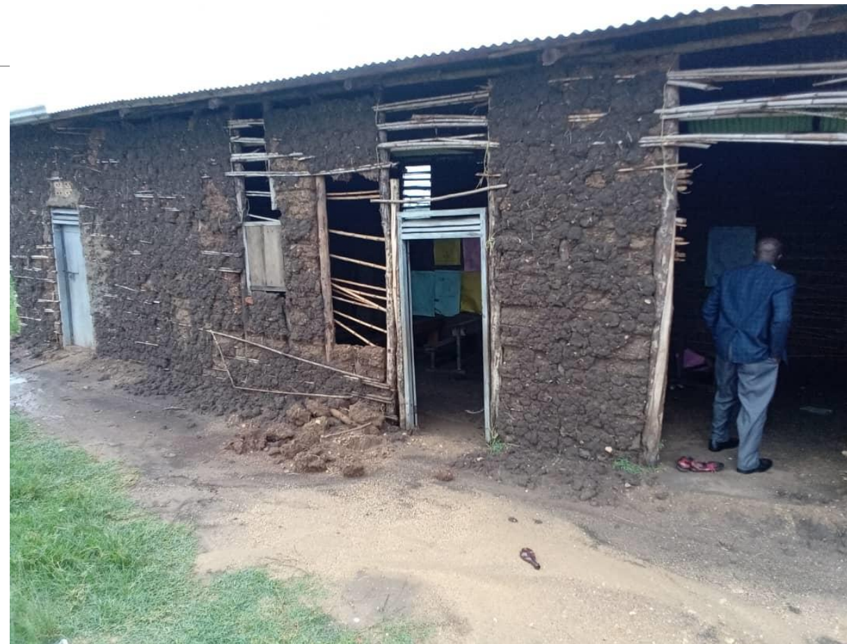
An in use condemned structure at Nyarurambi Primary School- Kitagwenda DLG
