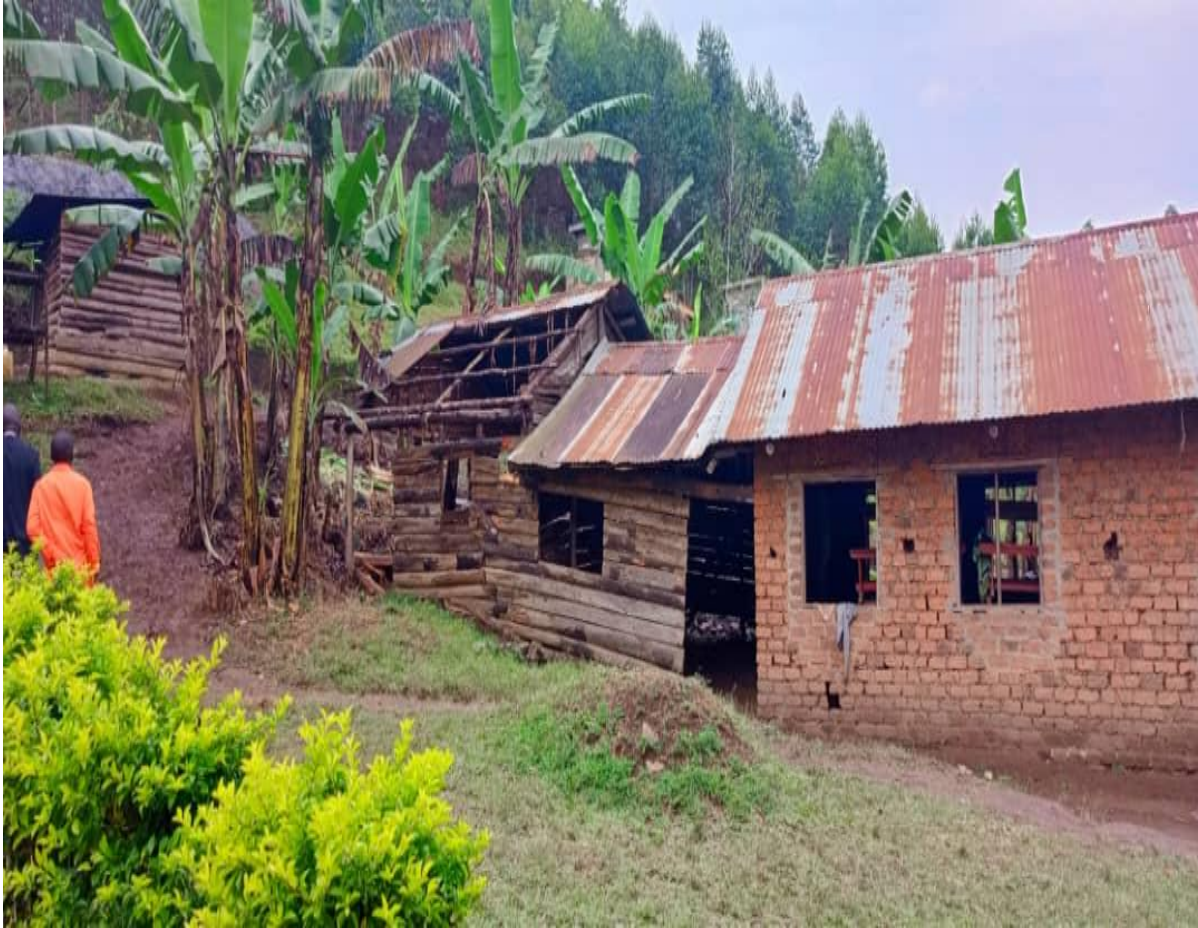
Poor state of classrooms at Butoha PS, Rubirizi DLG
