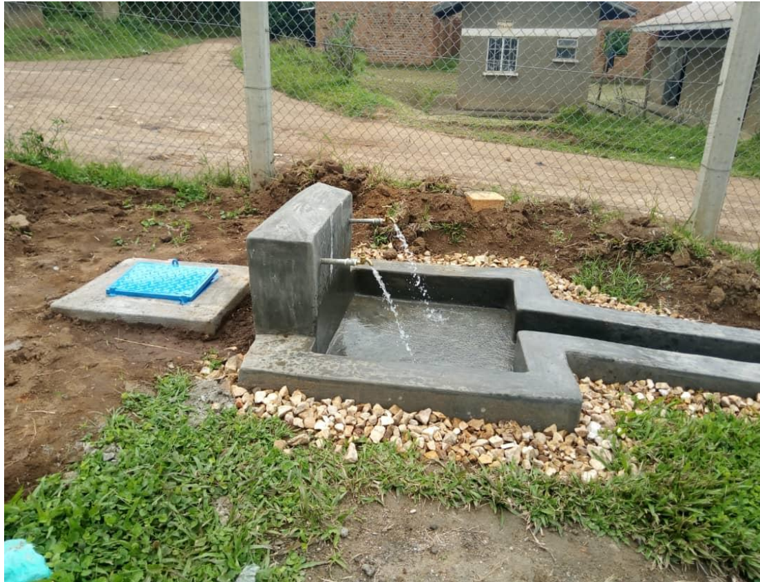
Provision of tap water to Muzira HC III- Sheema District
