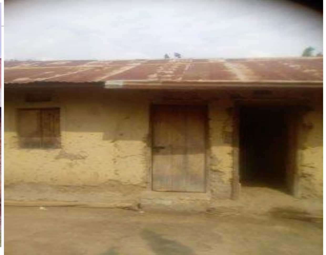
A dilapidated staff house at Kabutsye-Bataka PS, Sheema DLG
