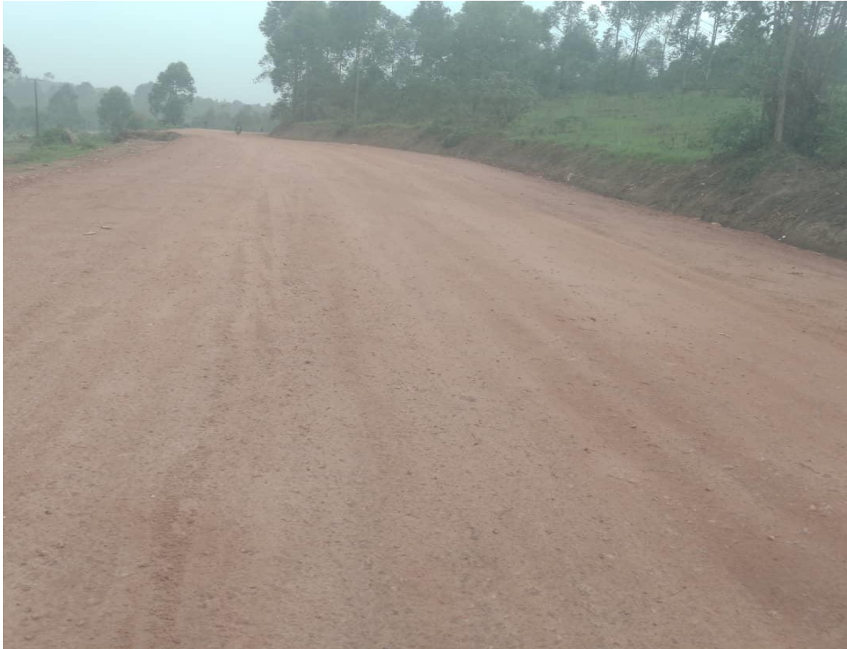
Expanding and gravelling st kagwa-kabagarambe road using road maintenance and transitional grant- Ishaka MC
