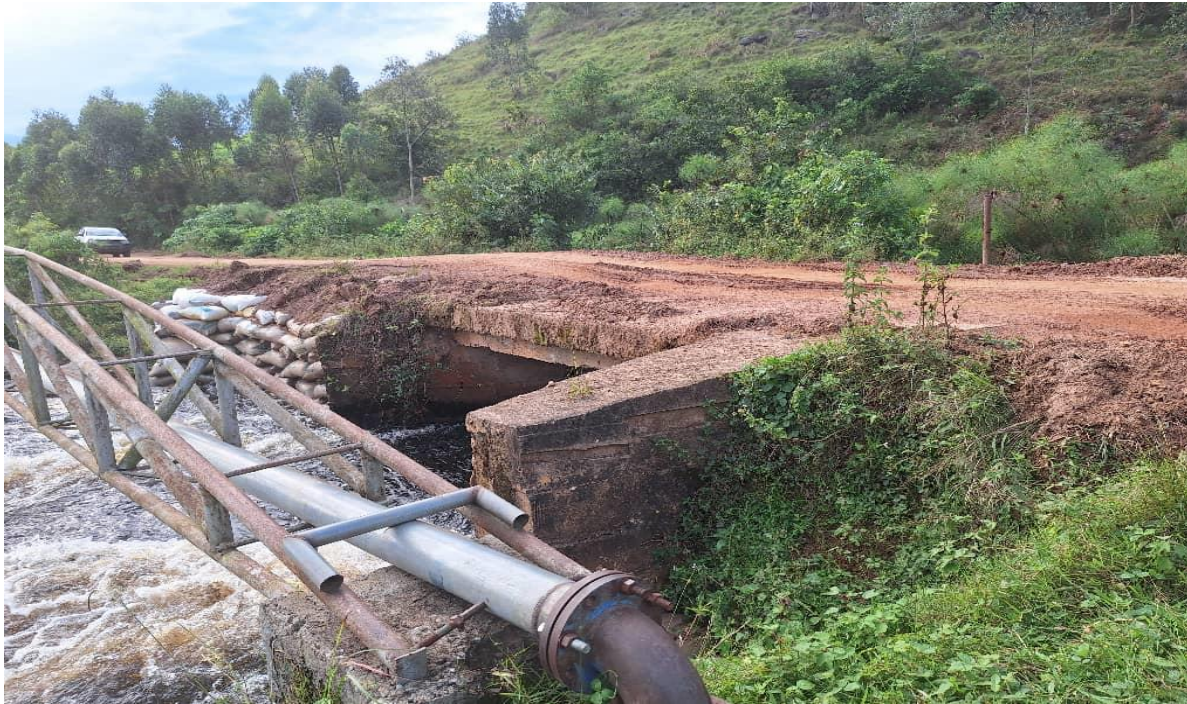
Poor state of Kyarwera bridge in Sheema district .
