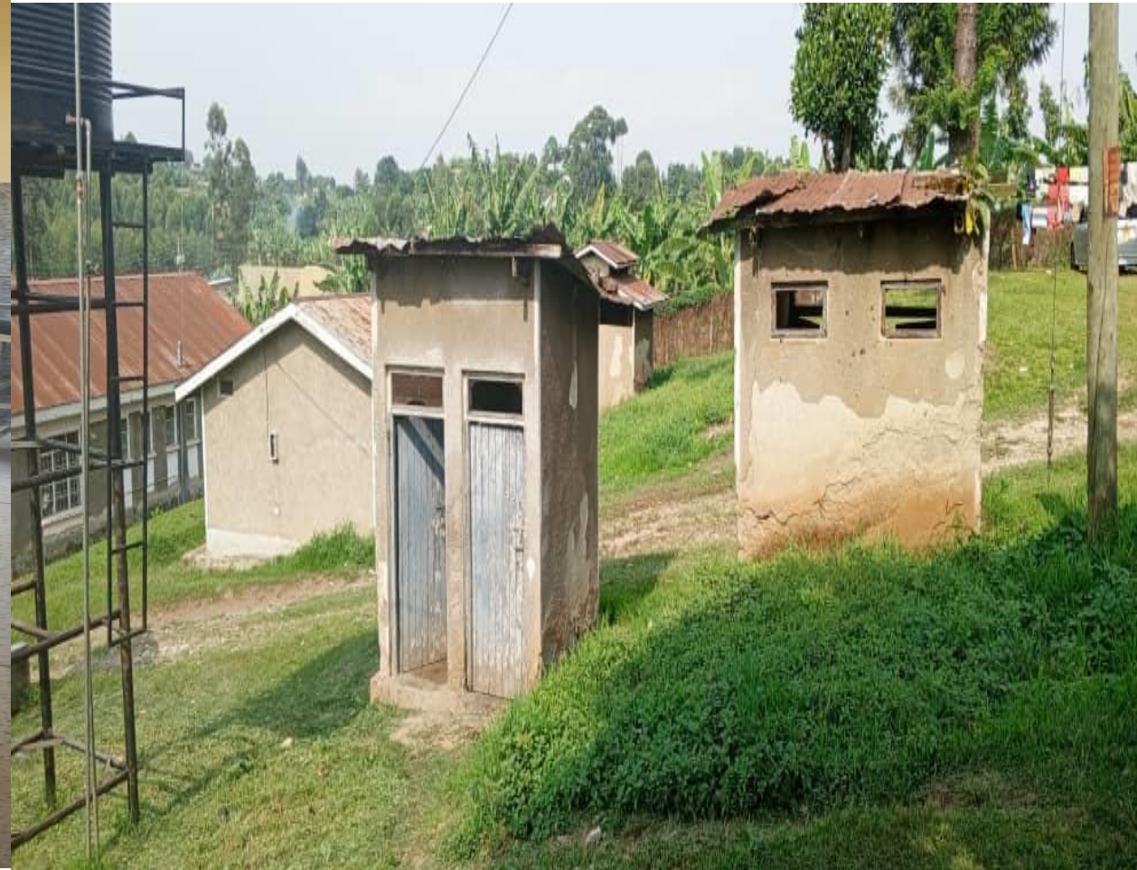
Dilapidated latrines at Rugazi H/CIV in Rubirizi DLG
