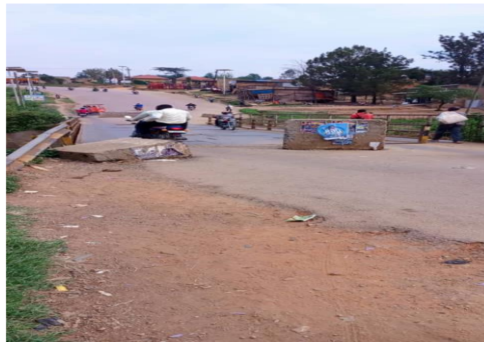
Katete bridge in Mbarara city that was closed due to its poor state
