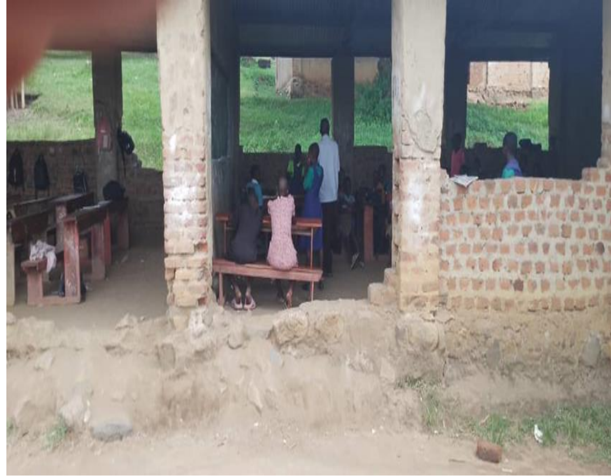
Incomplete classroom block at Bukangama ps – Bundibugyo DLG
