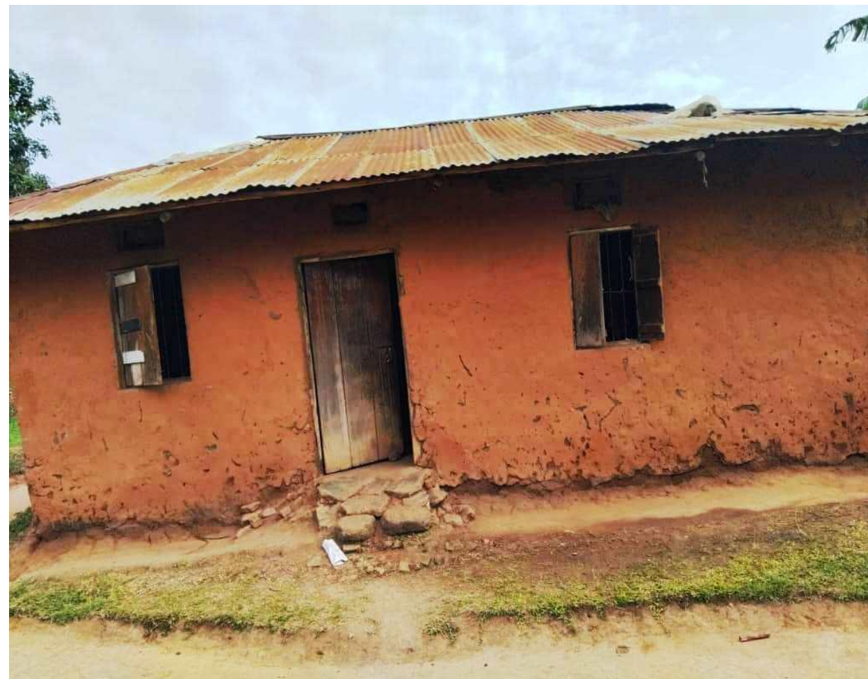
A dilapidated staff house at Mbarara Mixed P/S - Northern Division, Mbarara City
