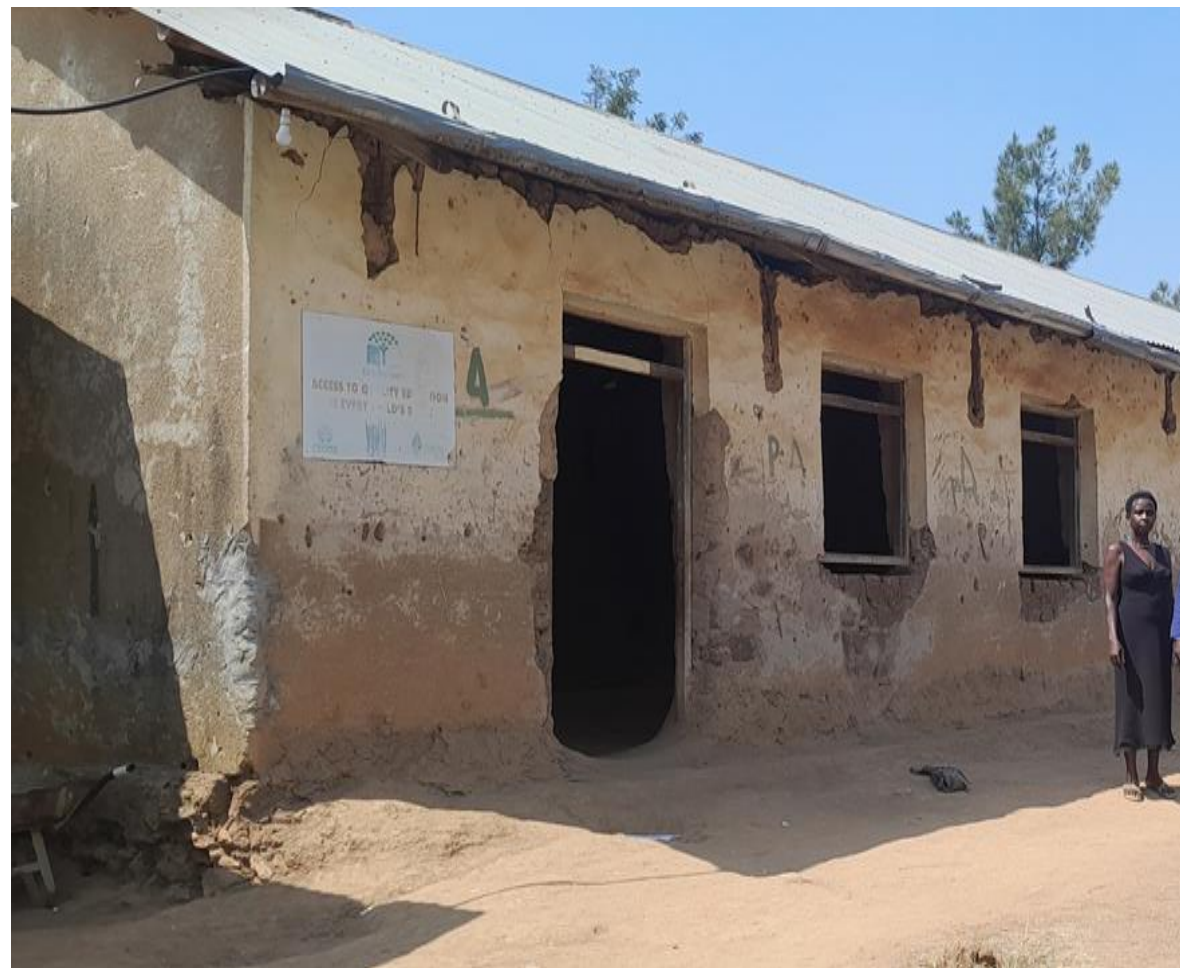
Dilapidated classroom block at Kishasha Primary school- Mbarara City
