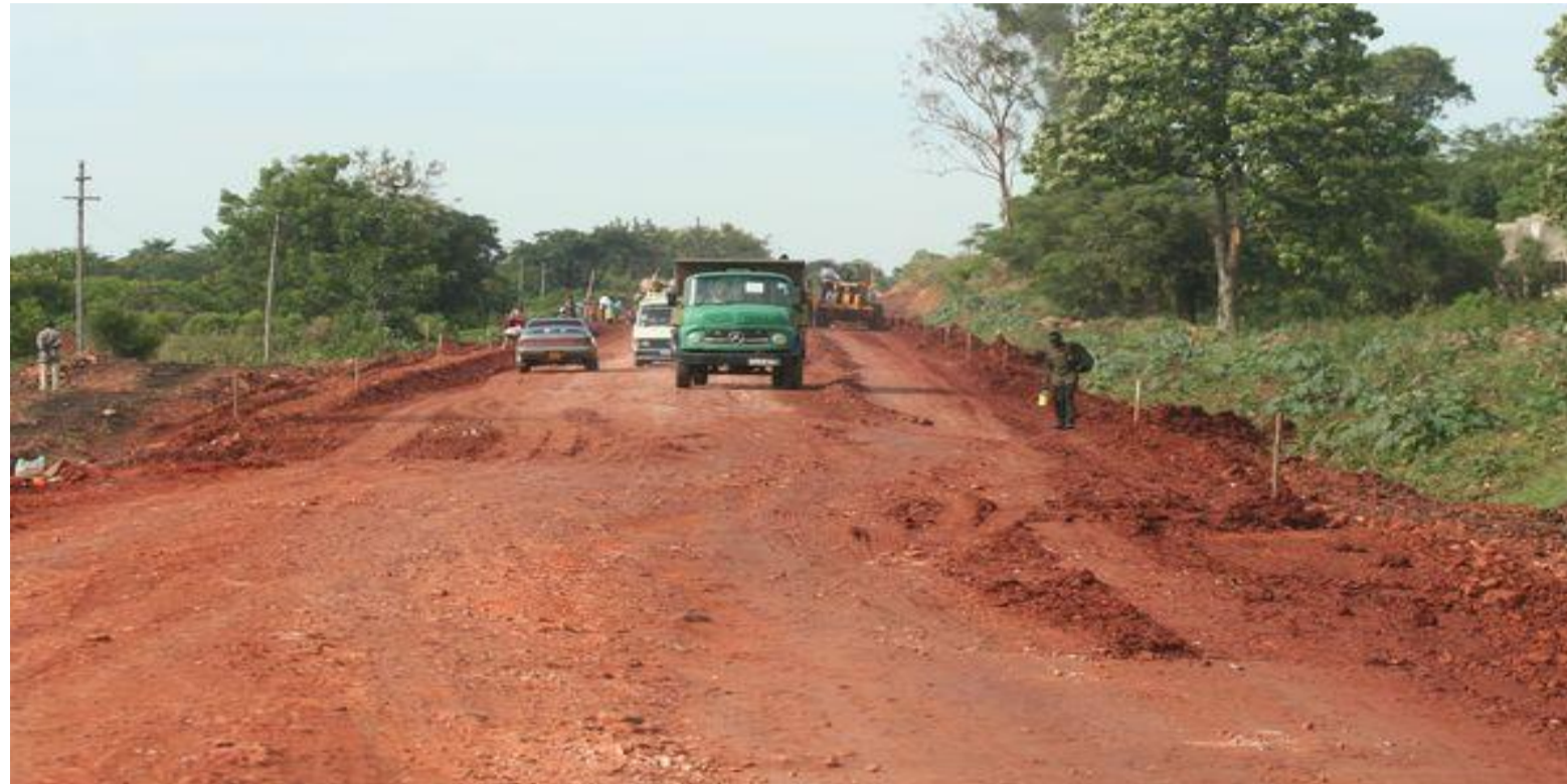
A road under construction. The parliamentary committee on Infrastructure will this month seek to know the status of roads which have been pending construction over the years. The committee will also seek to know the progress of the Standard Gauge Railway.
